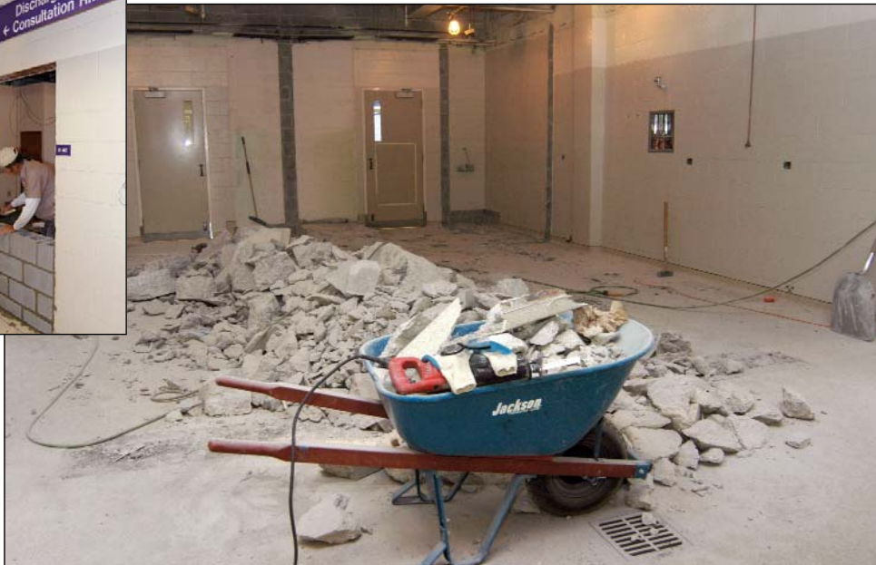
Left: Demolition is taking place for construction of the new ICU. This area was formally occupied by anesthesia, cardiology and exotics wards.
